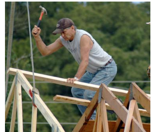
Smith, left, helps the Kenwood community with remodeling and replacing the roof on their community center. COURTESY PHOTO
